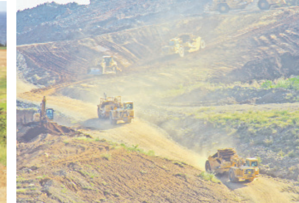
INCREASED COMPLEMENT of Motor Scrapers helps to speed up the work in the 2nd kilometer.
