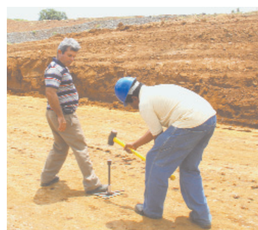
ENGINEERS PREPARING to test the compaction of the soil on the runway in the 1st kilometer.
