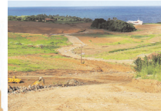
THE APRON, terminal building and runway areas being prepared in the 2nd kilometer.
