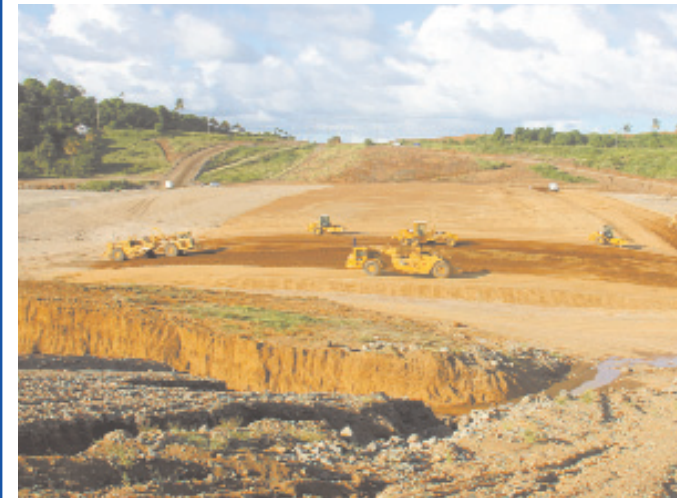
ANOTHER VIEW of this section of the runway in the 1st kilometer.
