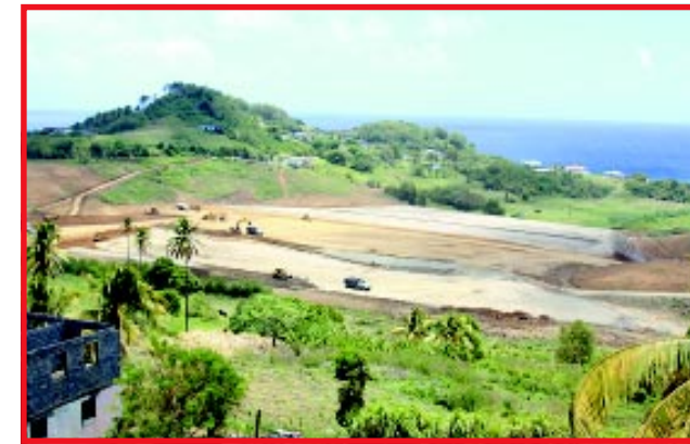
Another view of the earthworks. The soon to be developed Mt. Pleasant/Rawacou road is above
