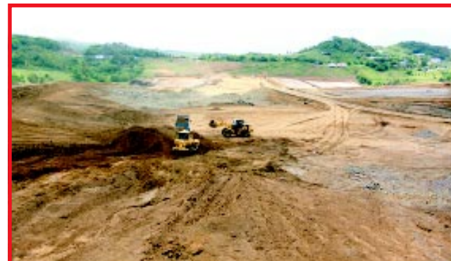
Excavation work, this soil is being used to help fill the embankment
