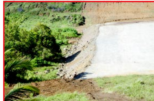
A section of the project site showing the height attained so far during the filling in process. They are expected to fill to a height of some 18 meters
