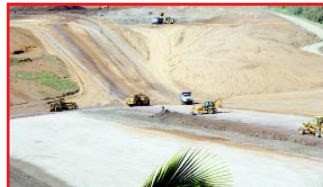
Heavy machinery and trucks engaged in the filling in process in the 1 st kilometer of the runway
