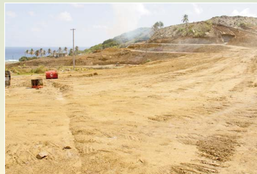
Work extends from Johnson Hill in the 1st kilometer into the 2nd kilometer.
