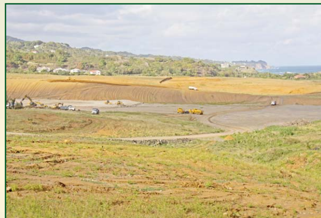
A view of the 2nd kilometer one week after the resumption of earthworks, following the Christmas break.
